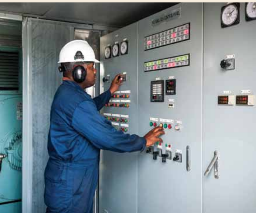
Nuestros técnicos monitorean el sistema 27/7 desde la sala de control. Our technicians monitor the system 24/7 from our control room.
