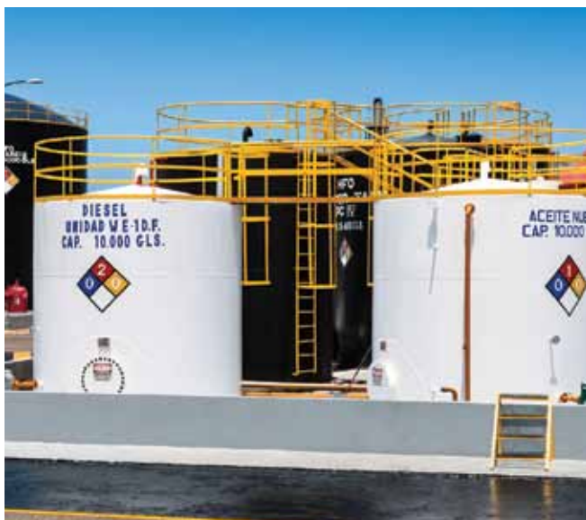
Tanques de combustible. Fuel oil tanks.
